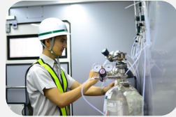
Continuous Emission Monitor Systems : CEMs
