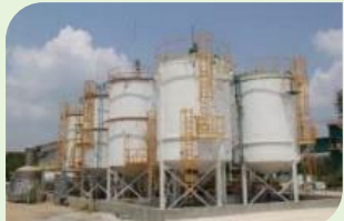
Liquid Treatment Plant
